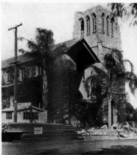
FIG. 13. TRINITY CHURCH, SHOWING DESTRUCTION OF END WALLS IN BASILICA TYPE BUILDING, STONE CONSTRUCTION
